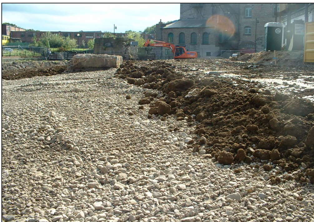
Former Byker City Farm. Placement of capillary break layer and clay cap.
