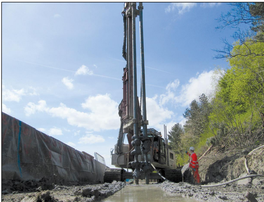
Installation of the soil mix barrier wall at St. Anthony's Tar Works
